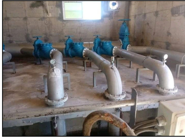
Figure 21 : Station de relevage
